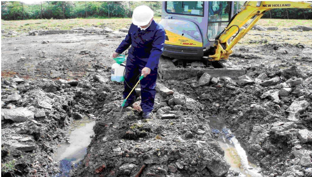
E-Safe™ being used in United Kingdom to treat hydrocarbon contaminated soil at a fueling depot in Lincolnshire.
